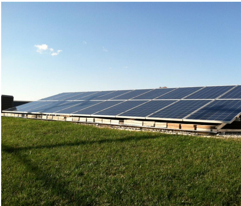
A 4.4 kw, 20-panel PV system on the roof of Prospect Solar's Sterling, VA office.
