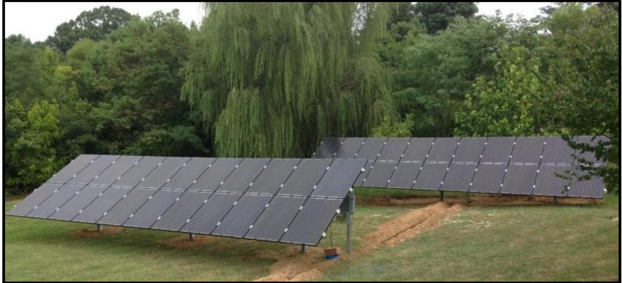
Figure 3. Ground-Mounted Commercial Solar PV System (12 KW) in Goochland County
