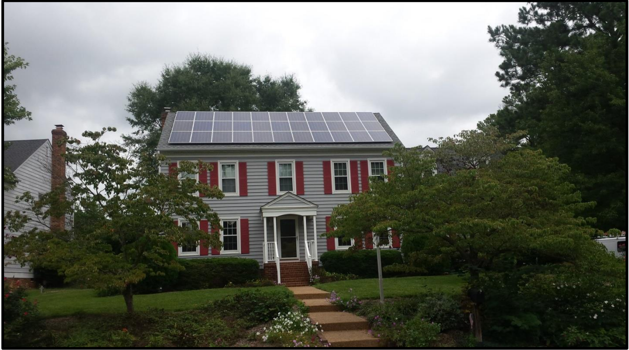
Figure 1. Rooftop Residential Solar PV System (8.25 KW) in Henrico County
