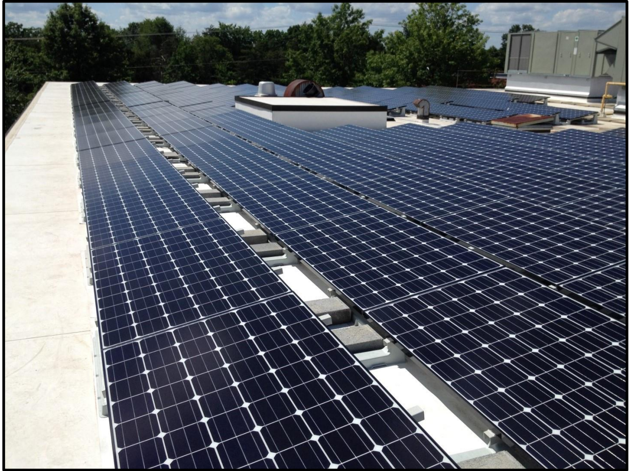
Figure 2. Rooftop Commercial Solar PV System (56 kW) in Chantilly
